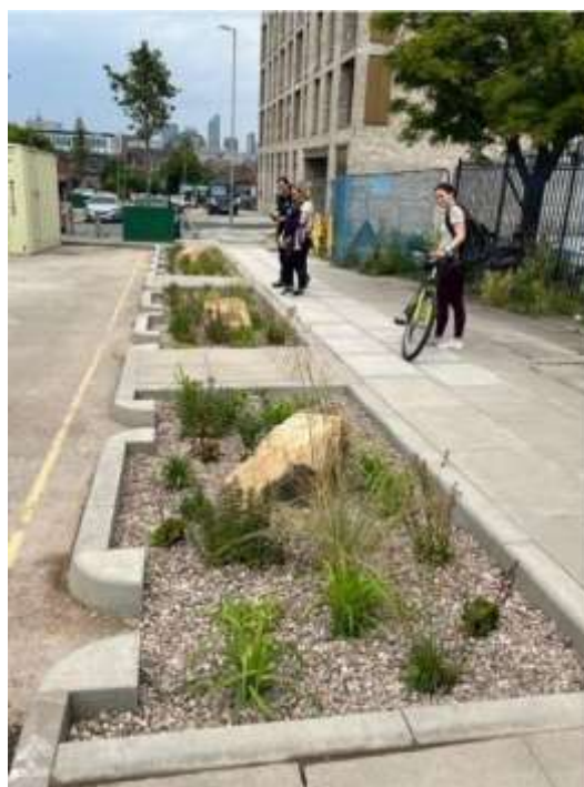
Completion of an urban raingarden Upper Pitt Street, Liverpool Source: Dr Juliet Staples, URBAN GreenUP, Liverpool City Council
